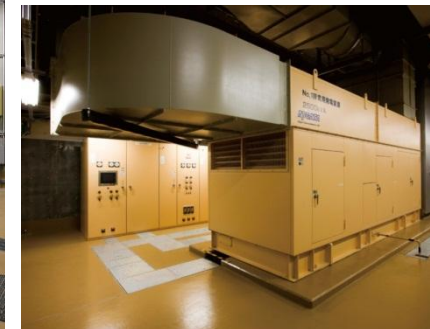
Emergency Power Generator
