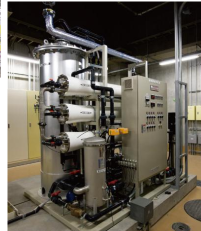
Emergency Pumping Facility
