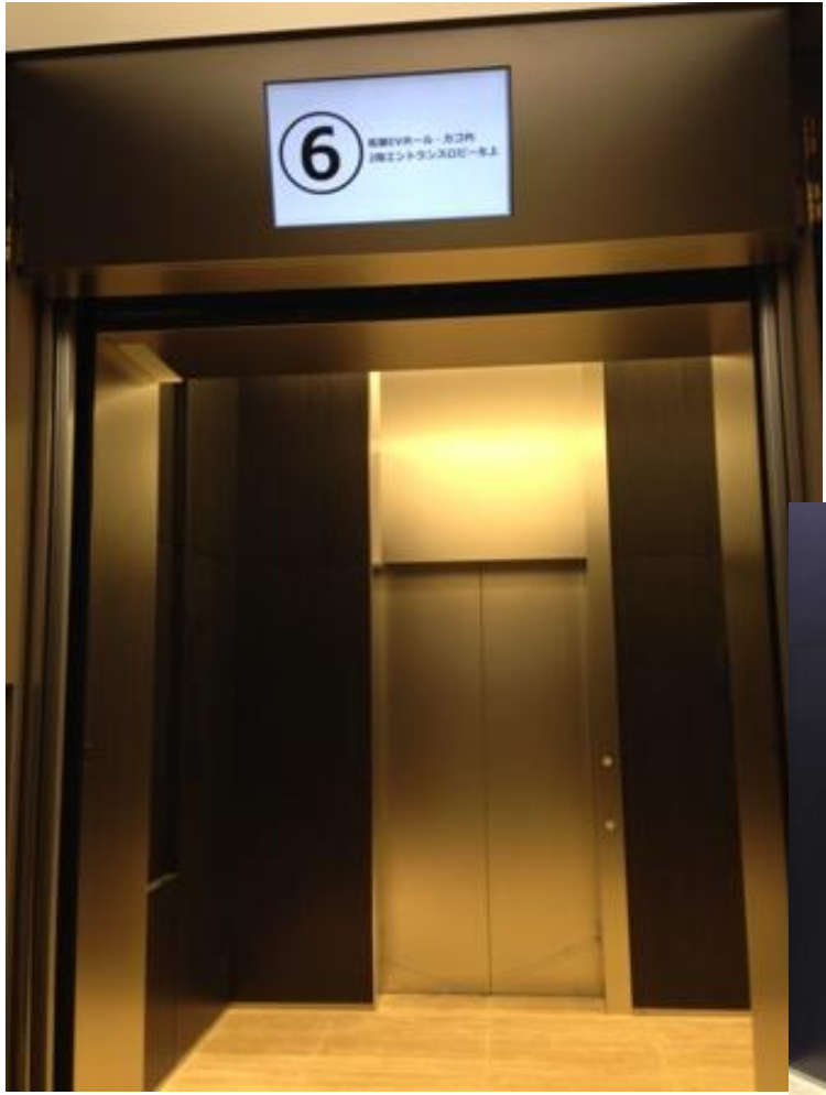
Monitor inside the elevator car
