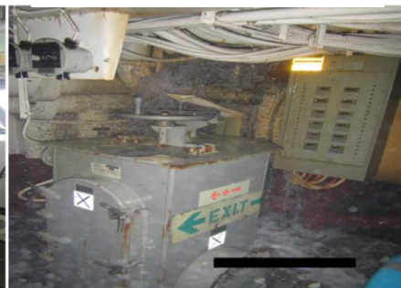
Inside damage ②
