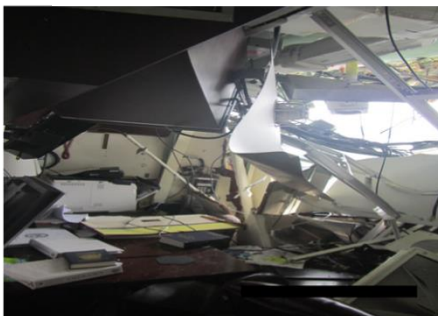
Inside damage ①
