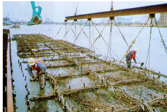
Lifting a fascine mattress in place (the next step being to put stones into the mattress)
