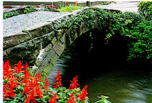
4) 73 Iguchi Bridge (Kikuyo-machi): completed toward the end of the Edo Period; mason: unknown; length: 10.75 m, width: 3.00 m, height: 2.65 m
