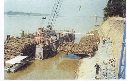
Installing foot-protection Soda-mattress in position with a crawler crane, mounted on the floating-dock barge
