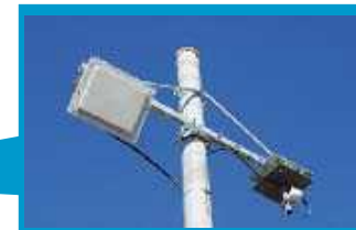
5.8 GHz DSRC roadside antenna
