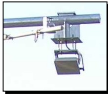
Roadside unit (DSRC antenna)
