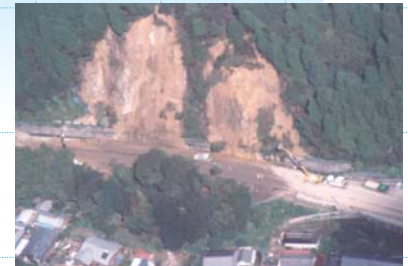
Damage to roads caused by heavy rain due to Typhoon No. 21 in 2004.
