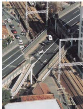
Damage to roads caused by the Great Hanshin-Awaji Earthquake in 1995
