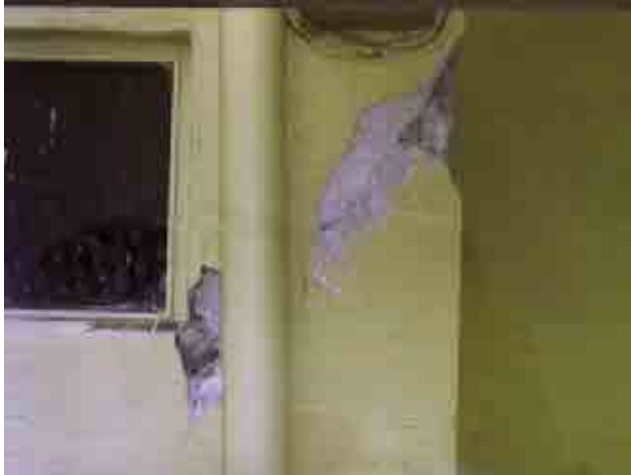
1) Wide shear cracks and local crush of cover concrete are observed at the upper part of column.
