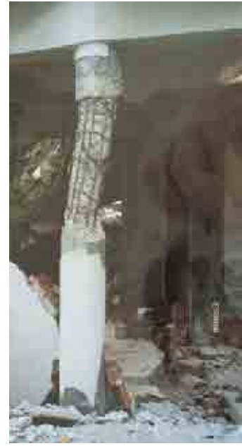
6) Crush of core concrete
