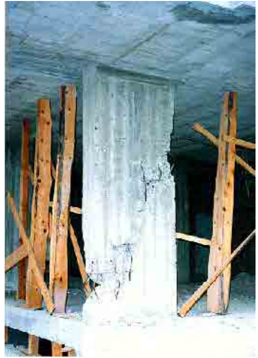
2) Buckling of reinforcing bars Crush of core concrete [2]
