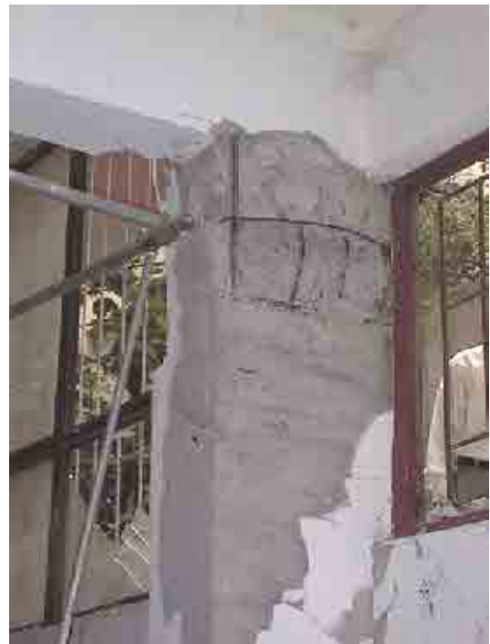
4) Buckling of reinforcing bars Crush of core concrete
