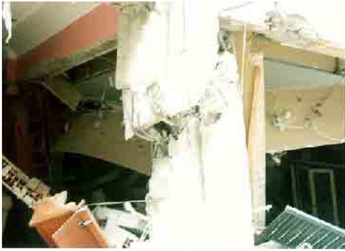
5) Visible settlement and/or inclination of floor [2]
