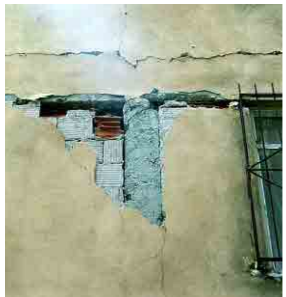
8) Big shear crack is observed at the top of the narrow face of column [2] .
