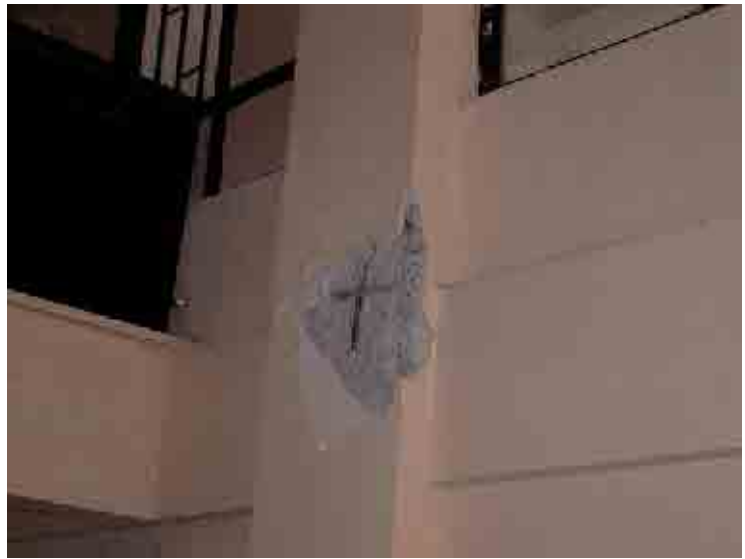
6) Mortar is fallen down. There was no cover concrete initially, so the reinforcing bars are exposed easily, but there is almost no cracks in concrete. So, damage rank is II
