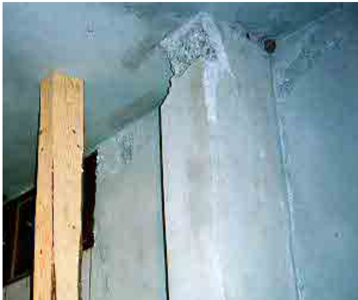
7) Big shear crack and spalling of cover concrete is observed at the top of column [2] .
