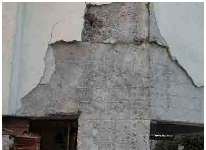
7) Visibly narrow shear crack and flexural crack occur in beam. No shear cracks are observed in the beam-column joint.
