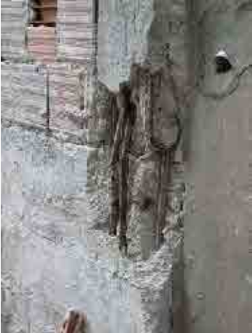
Concrete crush at the bottom of column and foundation beam-column joint.
