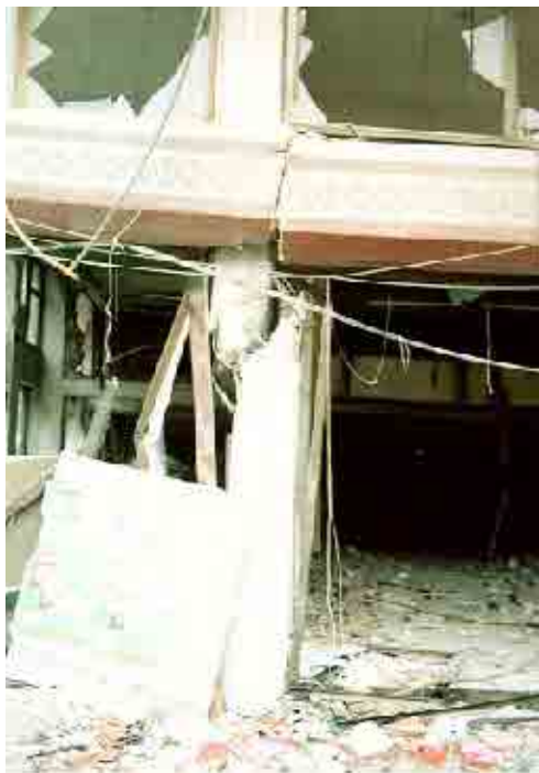
3) Buckling of reinforcing bars Visible settlement and/or inclination of floor [2]
