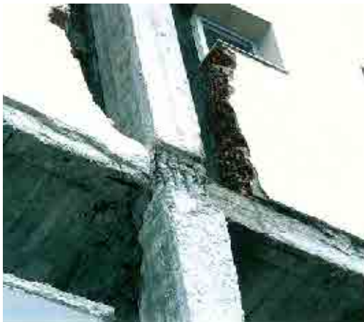
9) Heavy damage at beam-column joint [2]
