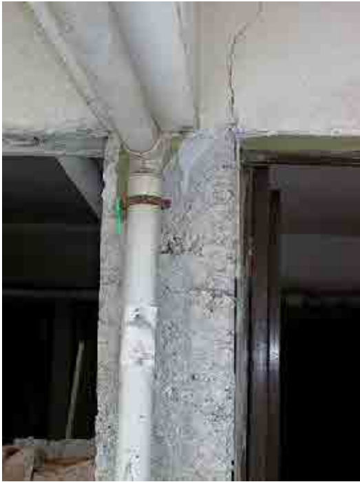
5) Visibly clear shear crack occurs at the top of the narrow face of the column.
