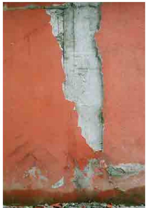
2) Mortar is separated and fallen down, and No shear cracks are observed [2] .
