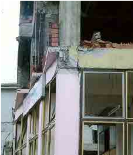
Diagonal shear cracks at the beam-column joint [2]
