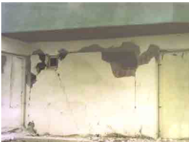
3) Big cracks, Massive Spalling of cover concrete and extensive exposure of reinforcing bars are observed [2] .
