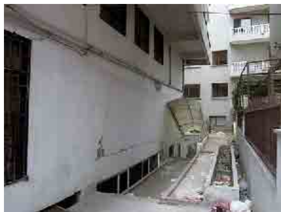
2) Rank B: Cracks observed but no out-of-plane deformation
