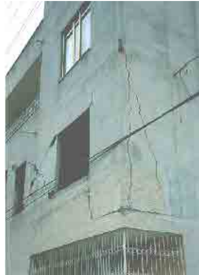
2) Rank C: Diagonal cracks observed and offset from RC frame [2]
