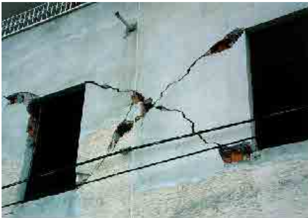
3) Rank C: Diagonal cracks observed [2]
