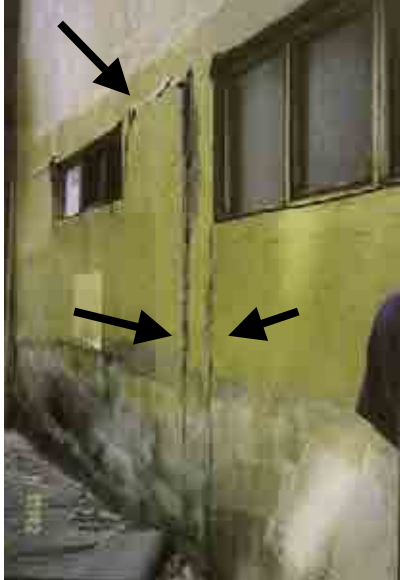
Cracks along interface between structural members (column and beam) and nonstructural wall are clearly observed.
