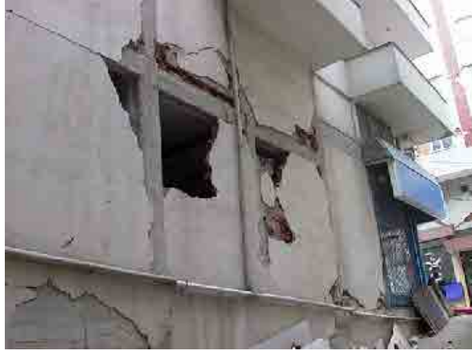
4) Rank C: Extensive cracks penetrated
