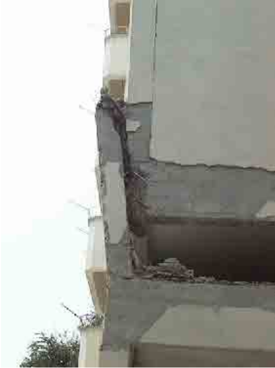
1) Visible settlement and/or inclination of floor
