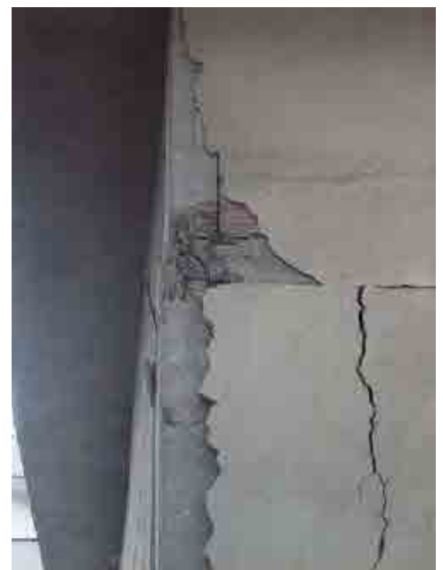
4) Diagonal shear crack is observed in beam-column joint.
