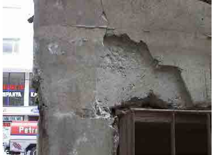
5) Only flexural cracks occur in beam
