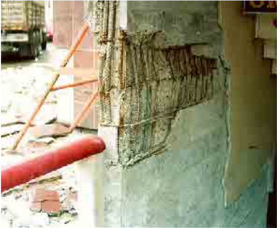
Tensile crack at the middle height of column [2]
