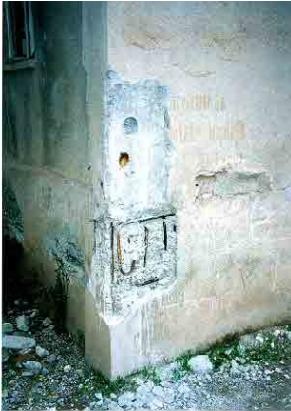
5) Massive Spalling of cover concrete and extensive exposure of reinforcing bars are observed, but buckling of the reinforcing bars is not observed [2] .
