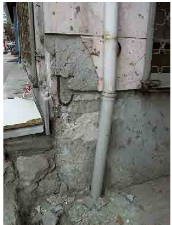
4) Evaluation of damage of this column is difficult. Spalling of cover concrete occurs at only corner. So, damage rank is II.
