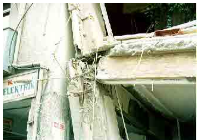
10) Crush of core concrete of beam-column joint [2]
