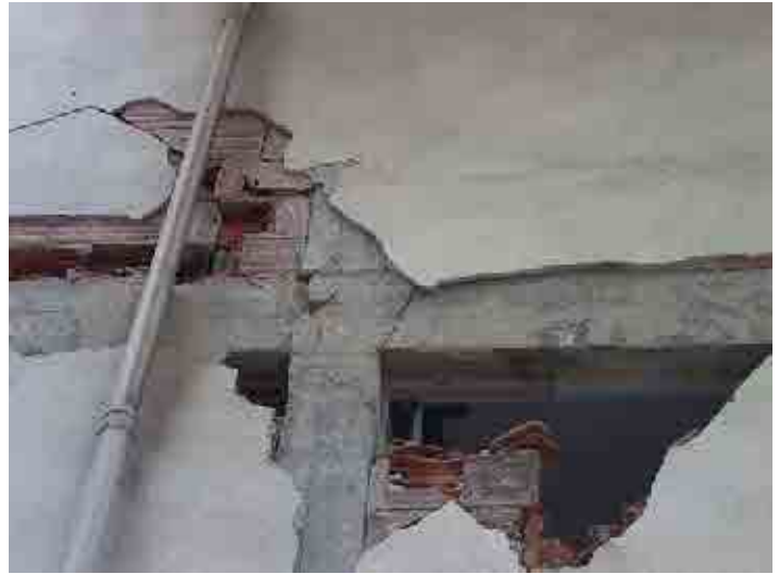
6) Wide shear crack and big flexural crack occur at beam end.
