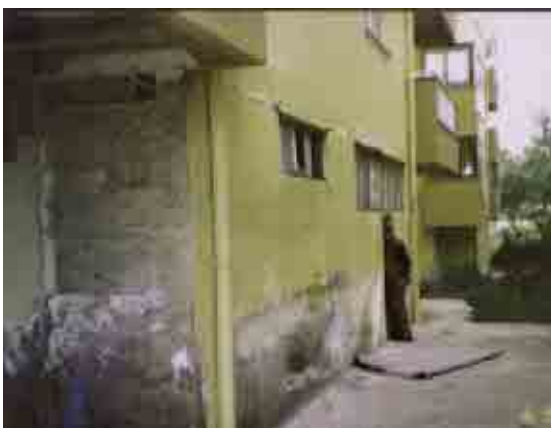
1) Rank A: Local crack and cracks at the boundary between wall and RC frame
