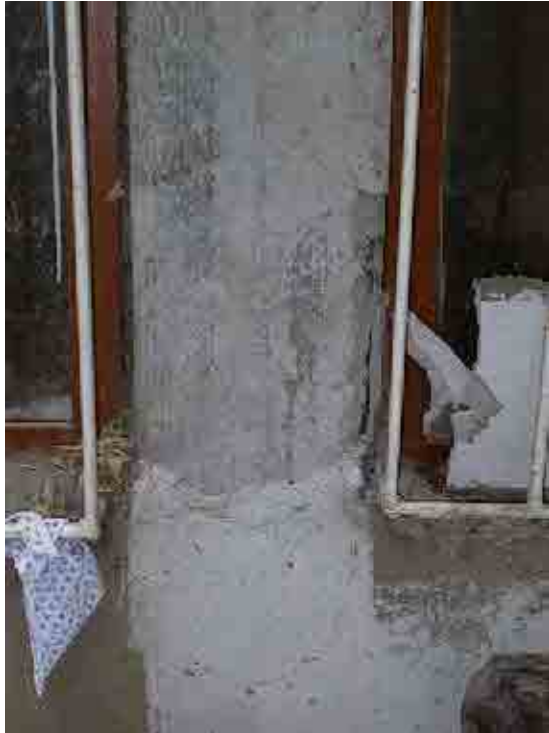
4) Corner cover concrete is spalled off. But shear cracks are not observed.
