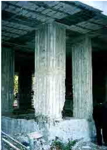
Concrete crush at the bottom of column [2]
