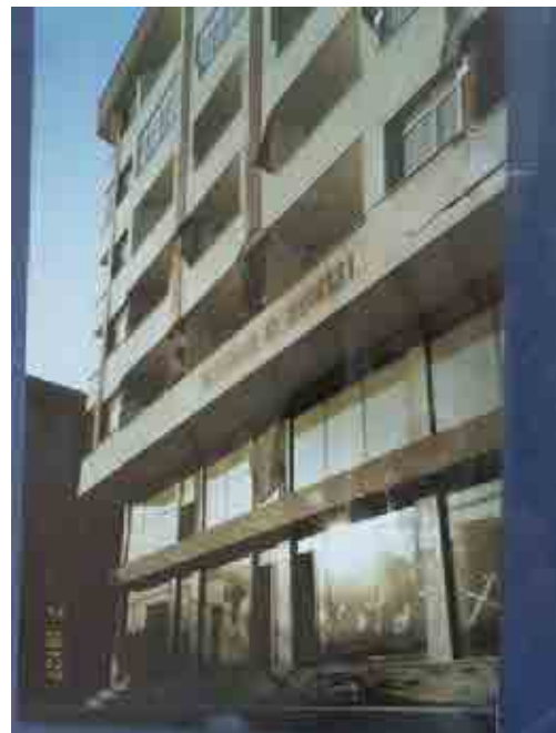
4) Rank C: Diagonal cracks observed in upper stories. Keeping out is needed near the building.
