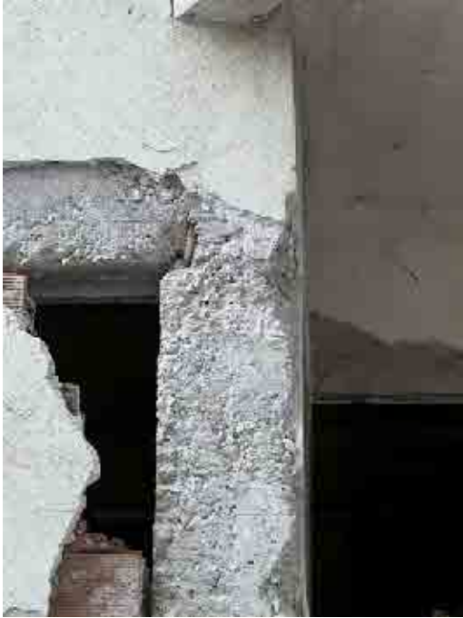
5) Construction quality is not so good. But almost no damage is observed in structural members.
