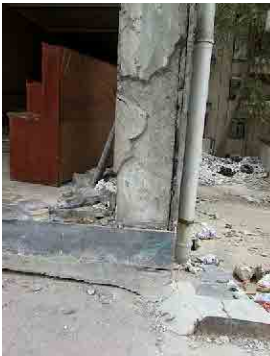
6) Corner cover concrete is spalled off. But shear cracks are not observed.
