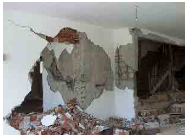
8) Buckling of reinforcing bars Crush of core concrete
