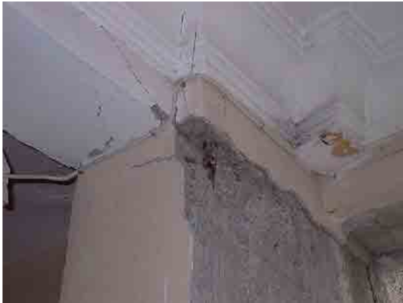
3) Wide flexural crack and local crush of cover concrete and small exposure of reinforcing bars are observed.
