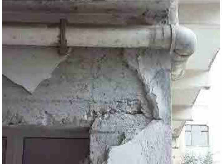
2) Construction joint is observed but negligible. Visible clear shear crack in the beam is observed.
