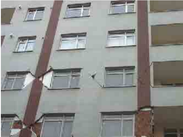
1) Rank C: Diagonal cracks observed
