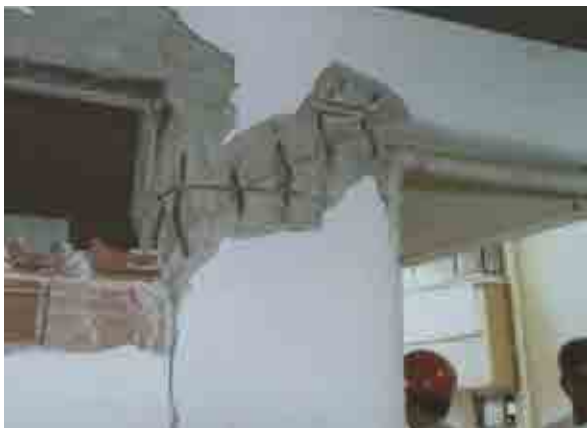
7) Buckling of reinforcing bars
