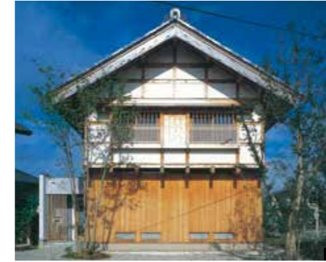
External wall finished with plaster coat at the top and boards on the bottom where the wall is exposed to rain.
