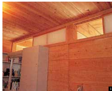
Ranma that closes to control ventilation
