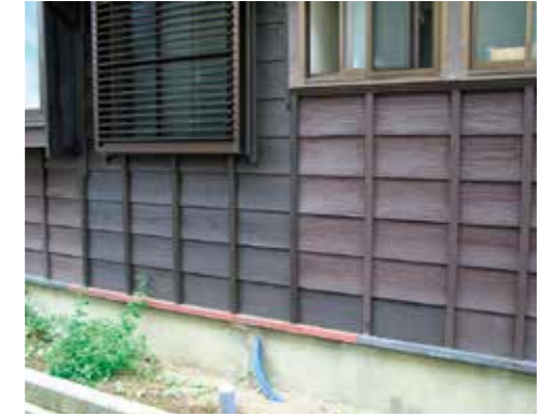
Partially replaced boarding and repainted so the repaired part is not conspicuous. (Washima, Niigata Prefecture)
