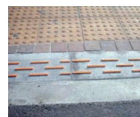
Edge structure of crosswalk which considers for the visually impaired, wheelchair users, etc.
