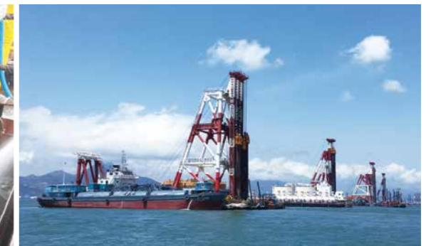
CDM改良船団による地盤改良施工状況 / Work being performed by fleet of CDM improvement vessels
