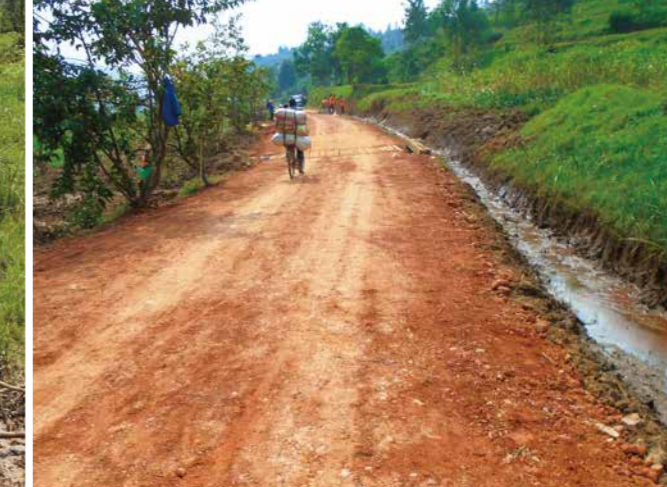
施工後スムーズに自転車で走行できる様子(ルワンダ) / Road after repair where one can ride a bicycle with ease (Rwanda)
