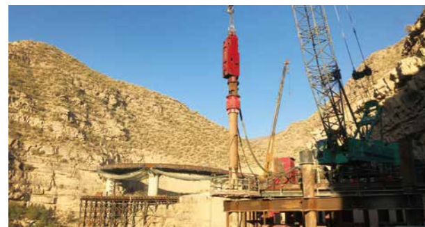
硬質岩盤への鋼管杭打設状況／Steel pipe driven into hard bedrock
