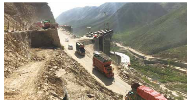
既存の道路機能を維持しながらの施工／Implementation of construction work while maintaining existing road functions
