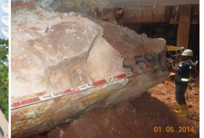
ベンクーレン駅掘削時に出現した巨大転石／ Gigantic boulders that emerged during the excavation work in Bencoolen Station
