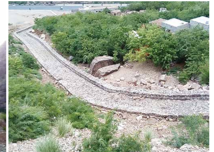
現地石材を用いた排水路 / Drainage canal using locally quarried building stone
