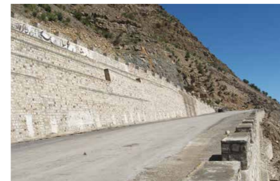
既存道路の石積み擁壁(建設前)／Masonry retaining walls for the existing road (before the construction work)
