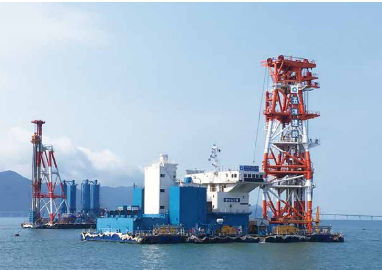
CDM改良船による大規模地盤改良工事/ Large-scale ground improvement work by CDM improvement vessels
