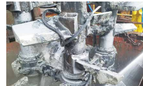
地盤改良機に巻きついた地中障害物の例 / Underground obstacle wrapped around the ground improvement device
