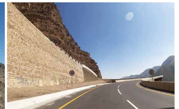
既設の石積み擁壁を有効活用した道路改良(建設後)／Road improvement making effective use of existing masonry retaining walls (after the construction work)
