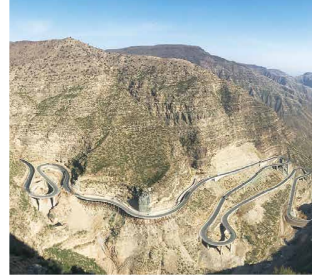
第1つづら折り区間の完成写真 / First zigzag section after the completion of the construction work
