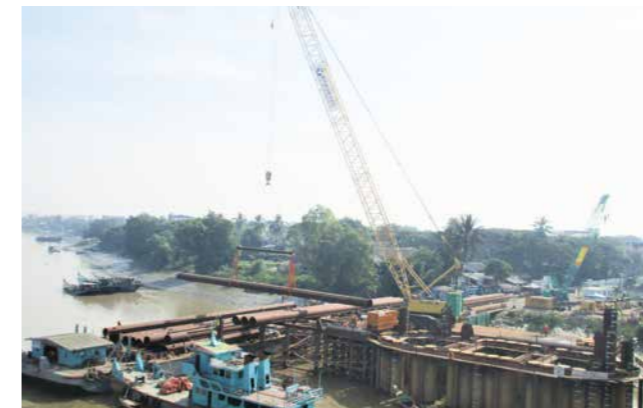
鋼管矢板の搬入と打設工事／ Delivery of steel pipe sheet piles and concrete placement
