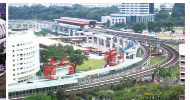
営業線近接工事のジュロンイースト駅改修工事 / Modification works to Jurong East Station that was close to operating lines
