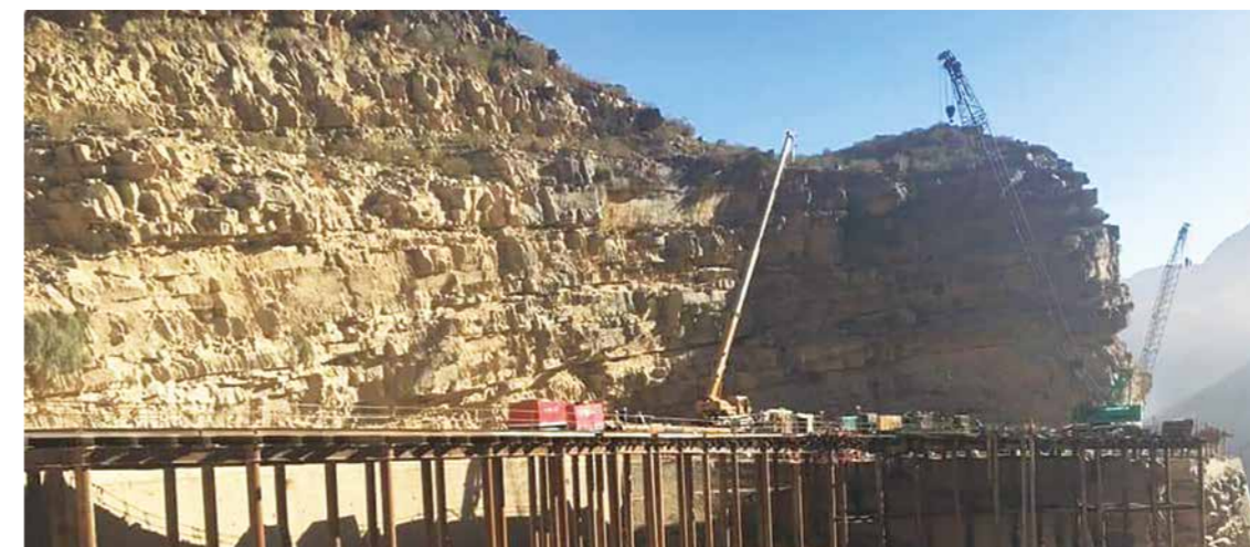
東西道路改修事業での施工管理の状況/Construction management of East-West Road Improvement Project
