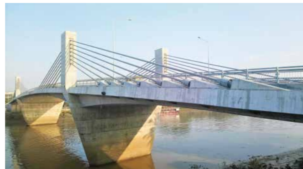
ケーブル定着部に制振装置を設置／ Installation of Vibration Damping Devices at Cable Anchorages
