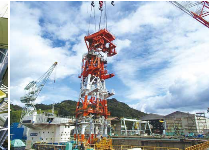
空頭制限対応のための檣の低頭改造状況 / Lowered scaffold developed in response to overhead space restrictions
