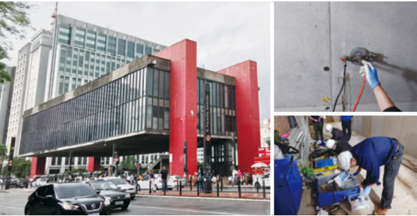
Repaired interior wall cracks that appeared in the new annex building of the São Paulo Museum of Art, a project contracted by Brazilian company RACIONAL.
