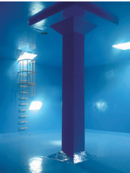
Inside of Distribution Reservoir The inside concrete surfaces were corrosion-protected using epoxy resin coating procured from Japan.
