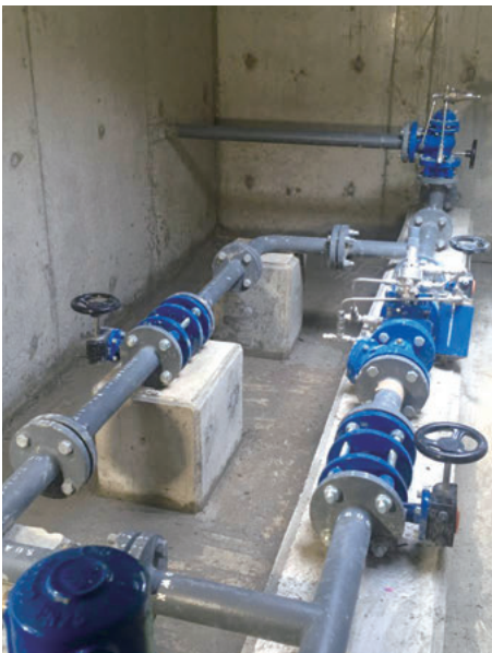
View of Pressure Reducing Valve Chamber A pressure reducing valve chamber was installed to maintain appropriate water pressure for each area following the conversion to a gravity-flow system.
