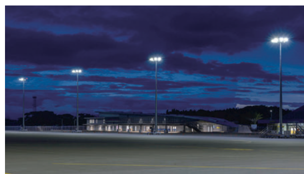
Apron lighting equipped with LED and a motorized raising/lowering system for easy maintenance
