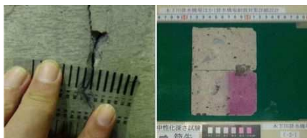
図-5 貫通ひび割れ1.2mm
