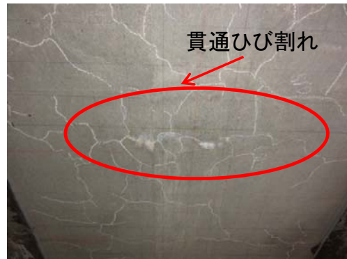
(a) No. 1 (貫通ひびわれ有り)
