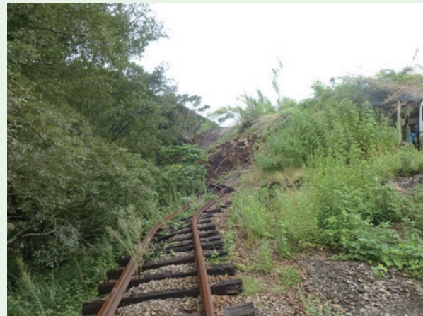
Damage on the Minami Aso Railway (between Tateno Station and Choyo Station)
