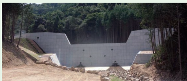
Closed-type Sabo dam
