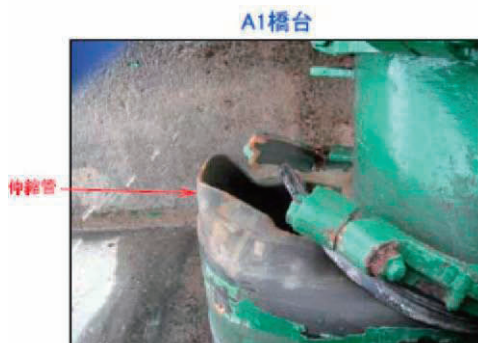
伸縮可撓管の破断
