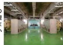
Water Purification Plant
