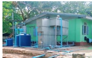
Water treatment system in Myanmar
