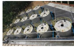
Sewage treatment system in China
