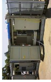
Industrial Plant Treatment (1.0 kg-O 3 /h)
