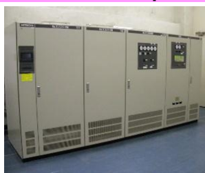
Uninterruptible power supplies
