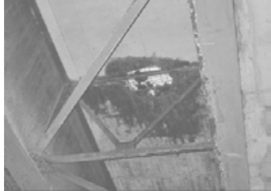
An reinforced concrete slab that has fallen out due to fatigue
