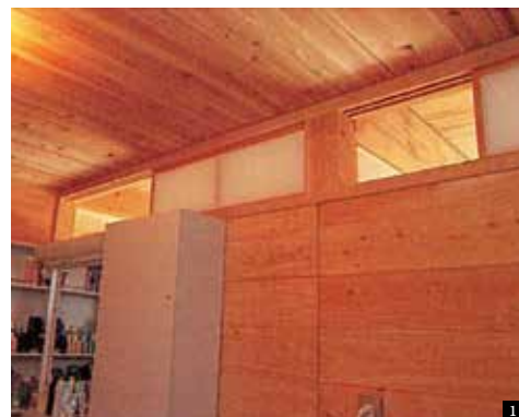
Ranma that closes to control ventilation
