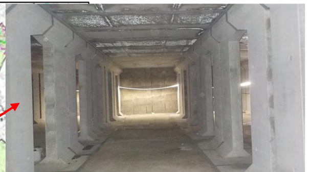
都雨水貯留槽 貯留量: 2,600m 3
