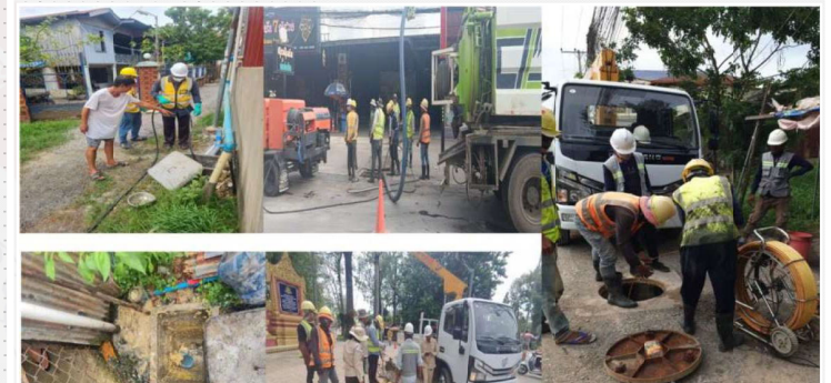
Blockage of Sewer pipe
