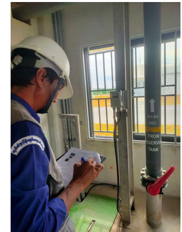
Checking the current flow of treated water flow
