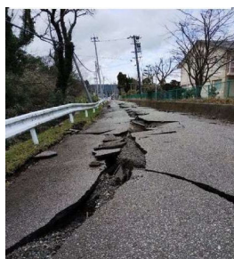
Severe damage to the sewer network caused by 2024 NOTO Earthquake
