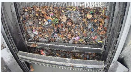
Operation during heavy rain (8 th Aug 2025)
