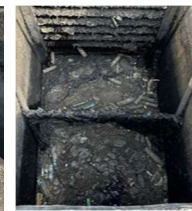
Sand & debris accumulation
