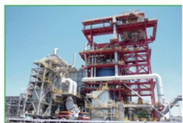
■ Coke Dry Quenching (CDQ) System
