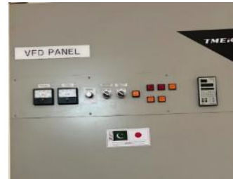
VFD (Inverter) Panel
