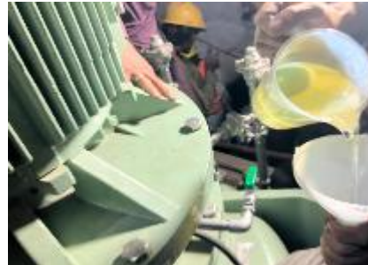
Lubrication oil filling process
