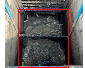
Sand & Debris accumulation
