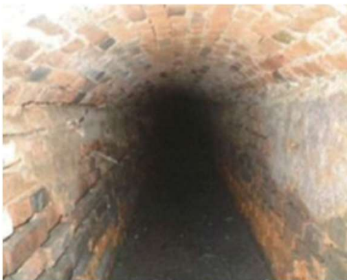
Host Pipe (Before)
