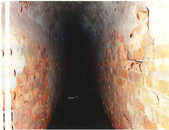
Host Pipe (Before)
