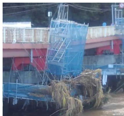
P2橋脚の沈下・傾斜
