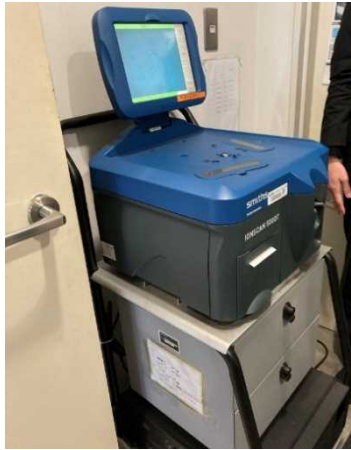
図 41 爆発物検査設備 (B. 国際貨物棟) 71
