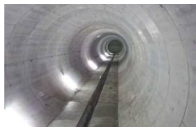
雨水貯留管(20,200m 3 )
