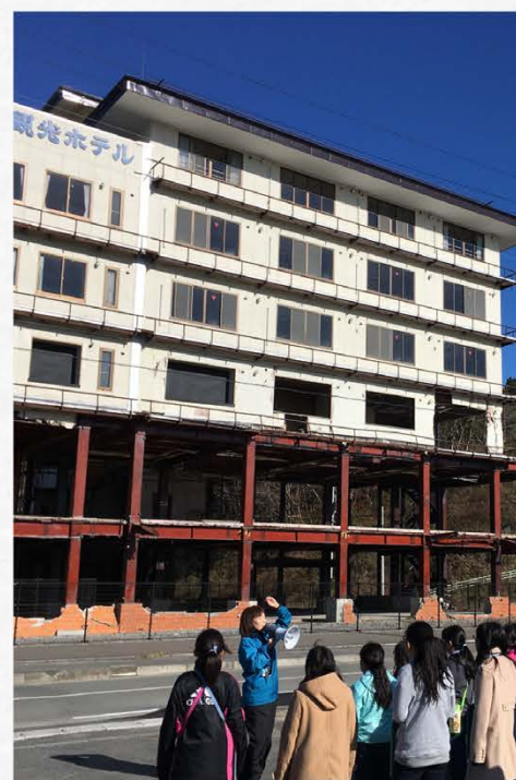
Active utilization of Taro Kanko Hotel, which was flooded and damaged up to the 4th floor
