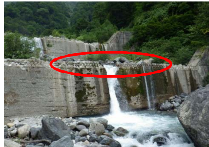
②水通し天端の摩耗
