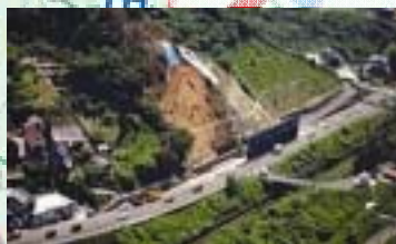
R9法面崩落(H18.7)
