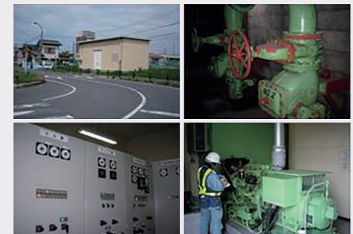
Example of drain pump
