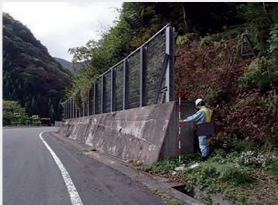
Rock falling protection fence
