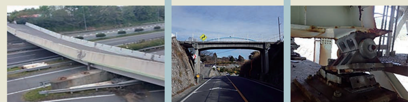
(1) Collapsed a rocking pier over Kyusyu Expressway (Prefectural road Ogawa-Kashima Line, Furoyo Daiichi Bridge) (2) Locally owned overpasses (have not been reinforced) (3) Damages on supports and main girders of a bridge (Heiryu Bridge, Oita Expressway)
