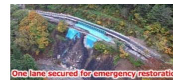
Heavy rain in August 2022 (National Highway 121, Yamagata Prefecture)
