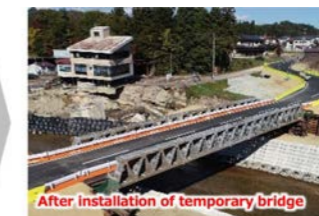
Heavy rain August 2022, Yamagata Prefectural Road 10 (Omaki Bridge)
