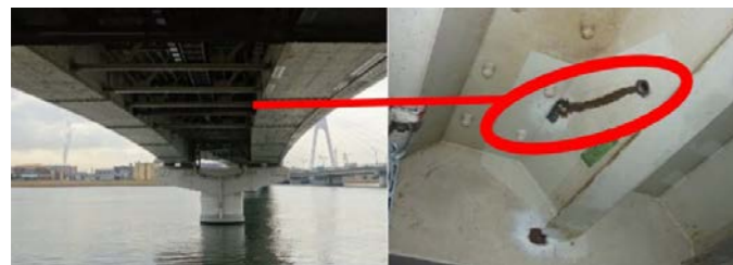
Numerous fatigue cracks in longitudinal ribs, etc.
