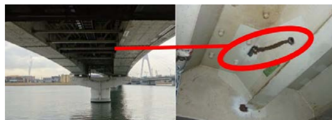
Numerous fatigue cracks in longitudinal ribs, etc.
