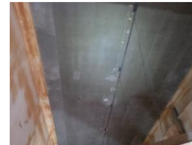
Bridge monitoring using optical fiber sensors
