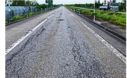
Asphalt pavement damage
