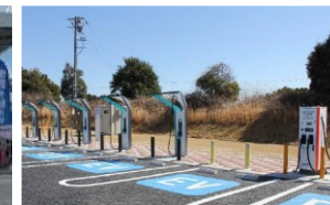
Promoting the installation of EV charging facilities
