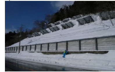
Example of Avalanche Countermeasures (Avalanche Barrier)
