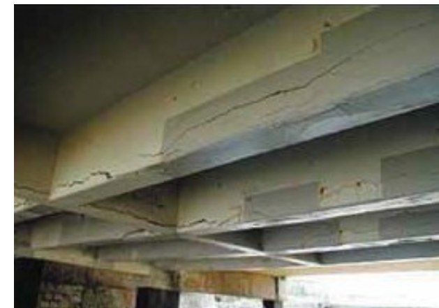
Deterioration due to an alkali aggregate reaction
