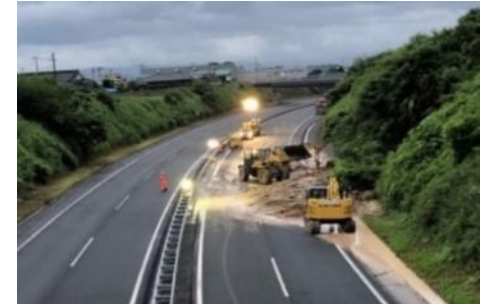
Utilize the undamaged two lanes to maintain traffic functionality
