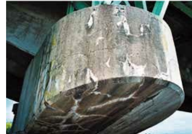
Deterioration due to salt damage
