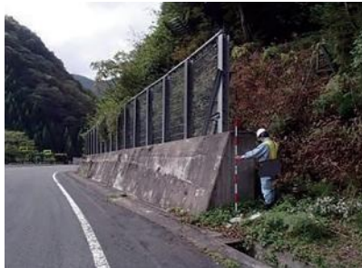
Rock falling protection fence
