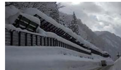
Snow protection work (Hokuriku Regional Development Bureau)
