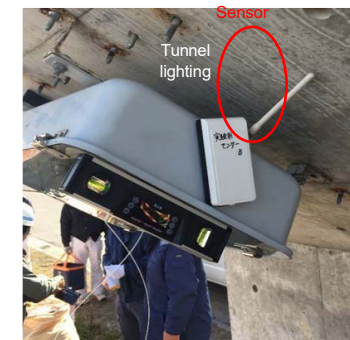
Anomaly monitoring sensors for tunnel accessories
