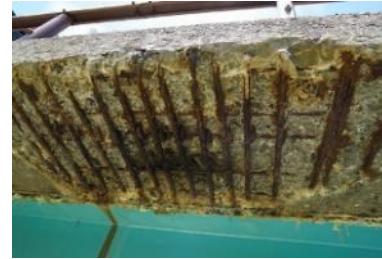
Exposed reinforcement in floor slabs
