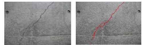
Fig.4 Crack detection results
