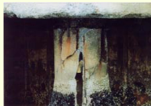
岸壁PC杭の亀裂
