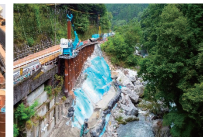
Rain-induced Road retaining wall failure (Japan) → Construction in the confined and elevated site
