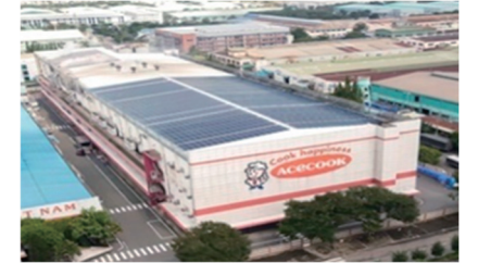
ACECOOK VIETNAM Solar power generation equipment
