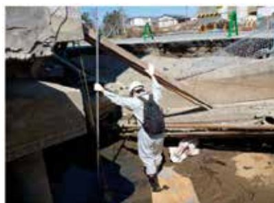
▲ 官庁施設の被災状況調査 Survey on a State of Damage to Government Buildings
